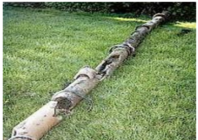
Failed section of the wastewater collection system
