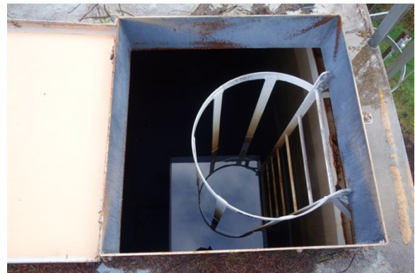
(#24) Roof Access Hatch Interior and Interior Ladder with Ladder Cage
