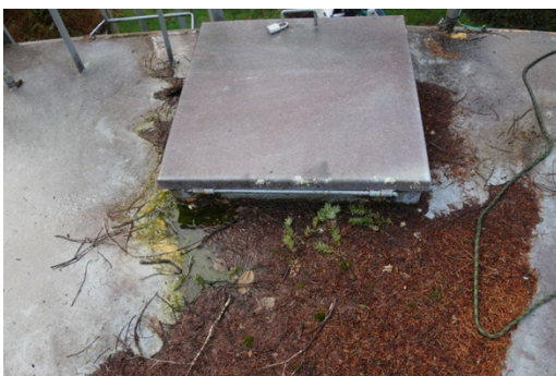
(#45) Before Confined Space Entry Placard Installed on Roof Access Hatch
