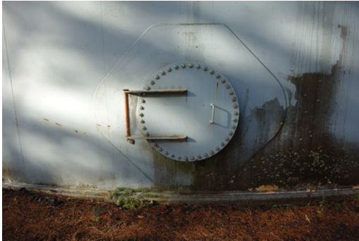
(#43) Before Confined Space Entry Placard Installed on Manway
