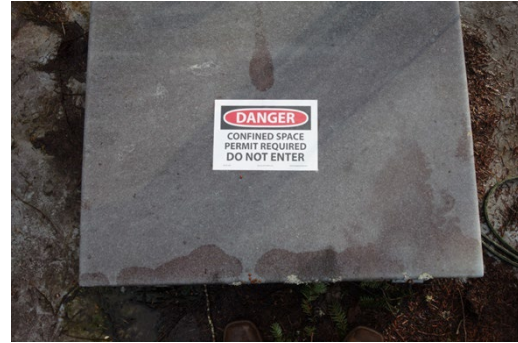
(#46) After Confined Space Entry Placard Installed on Roof Access Hatch
