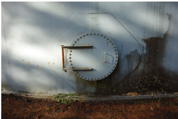
(#3) Manway and Exterior Coating Condition #2
