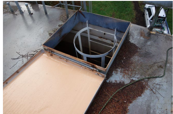
(#23) Roof Access Hatch Missing Gasket
