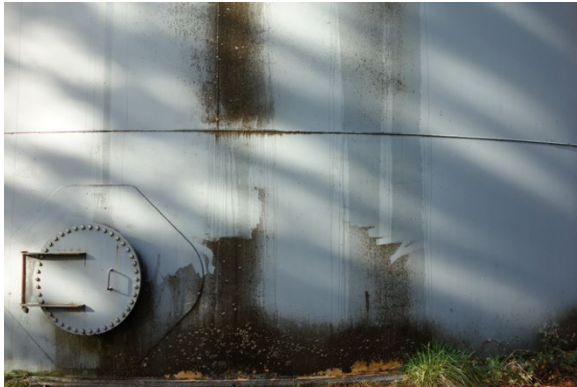
(#2) Manway and Exterior Coating Condition #1
