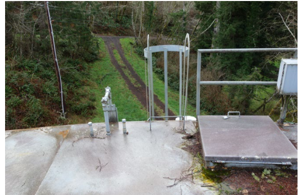
(#17) Exterior Ladder and Ladder Cage, Roof Penetrations, Roof Access Hatch, Exterior Electrical, and Roof Coating Condition
